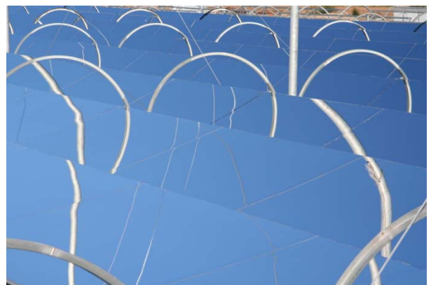
Steel-backed mirrors track the sun, heating water to create reliable, low-cost steam.
